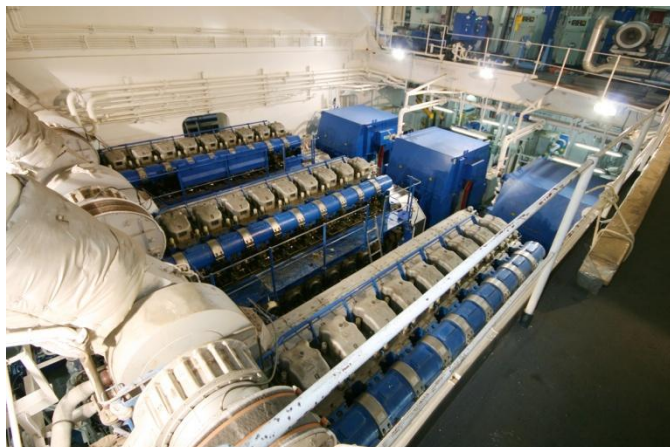
MAN Diesel 32/40 engines pictured within the Simon Stevin's engine room
