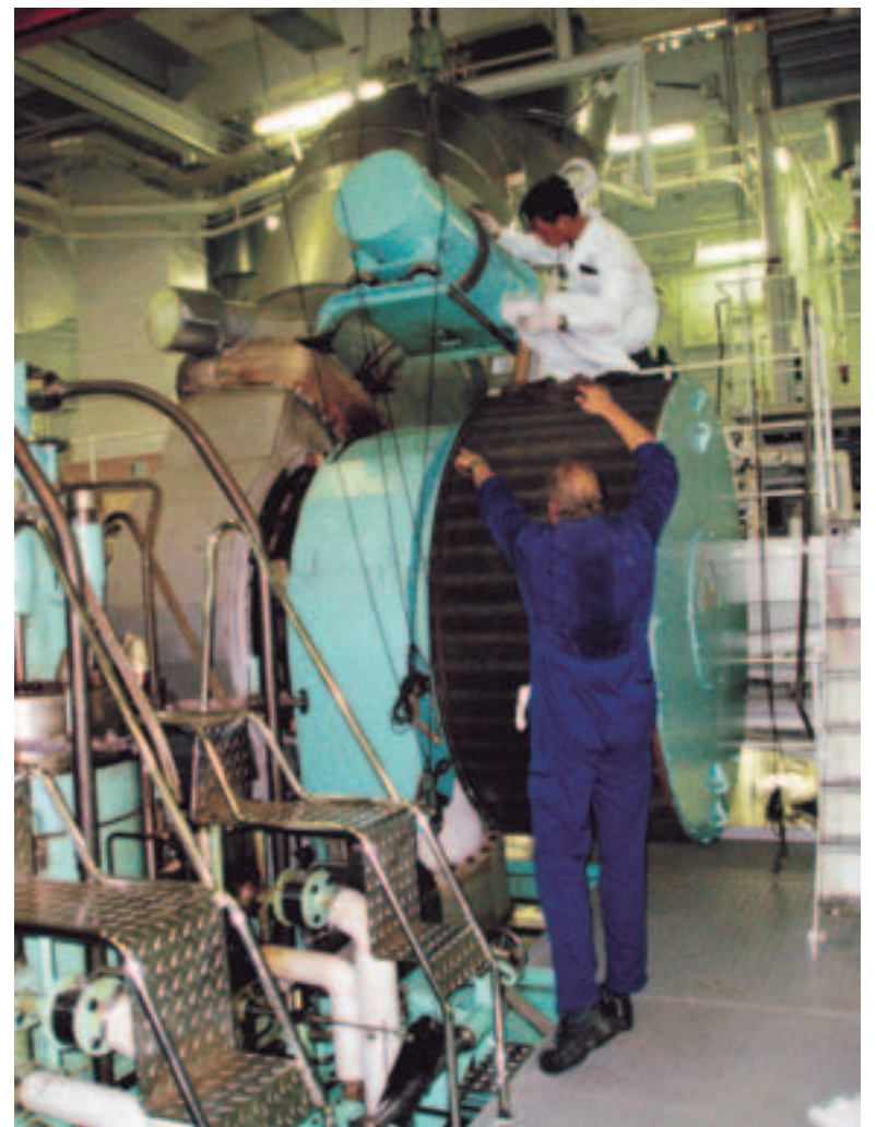
Inspection and assessment of the TCA turbocharger's condition.
