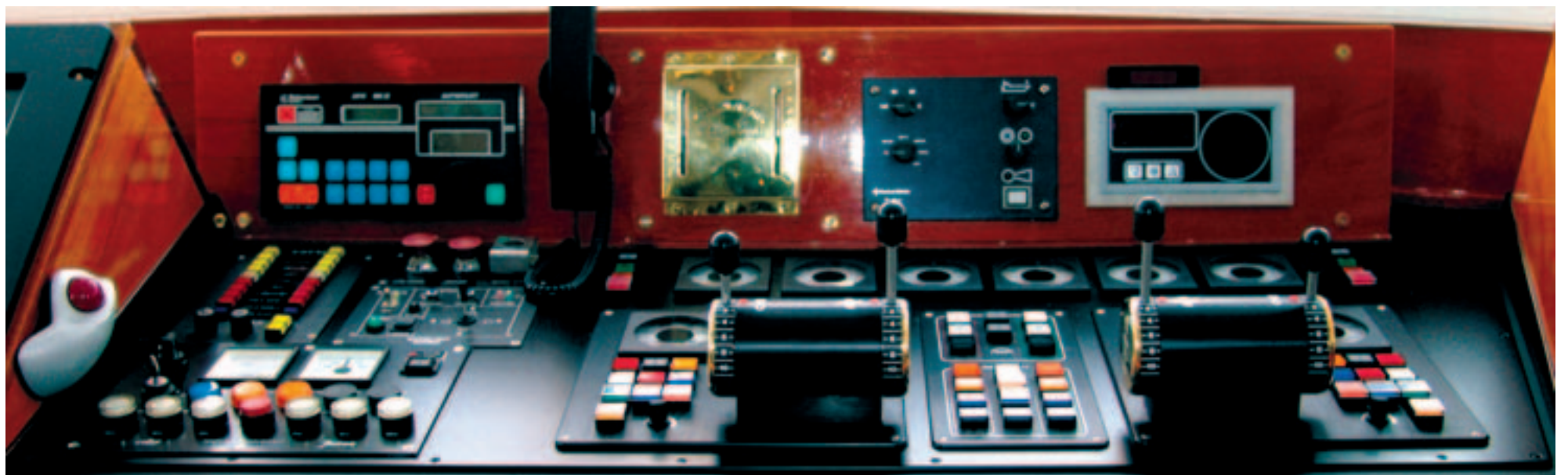
The bridge main control panel
