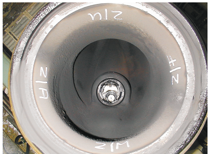
Clean exhaust valve duct with slide fuel valve 890 hours after installation
