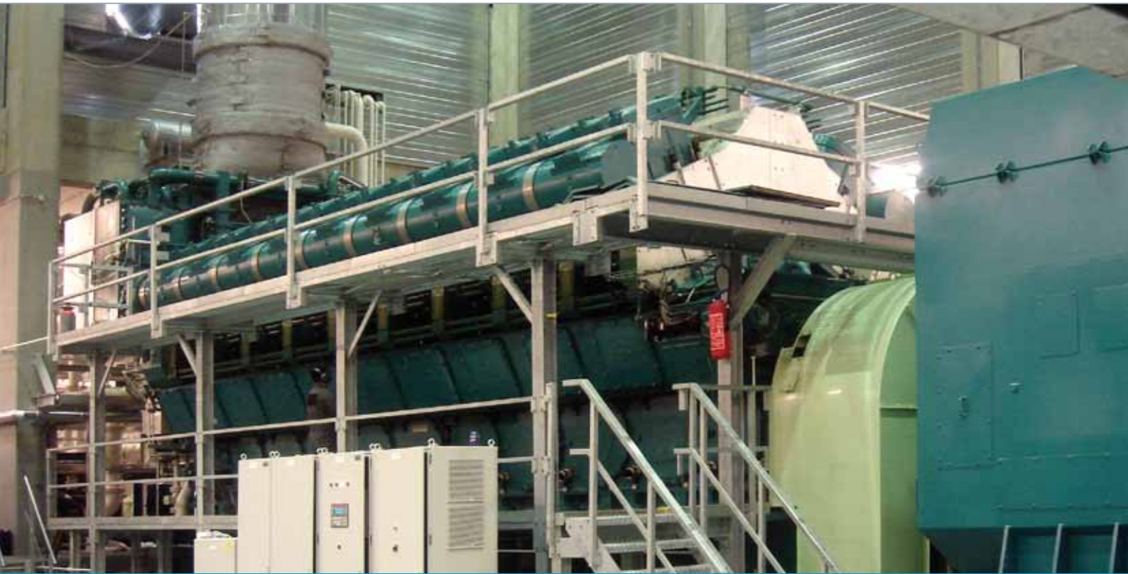
The 17.7 MW rated type 18V48/60 engine at the Electrawinds co-gen plant in Mouscron, Belgium
