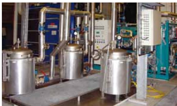
Fuel is processed by heating and 3-stages of progressively fine filtration
